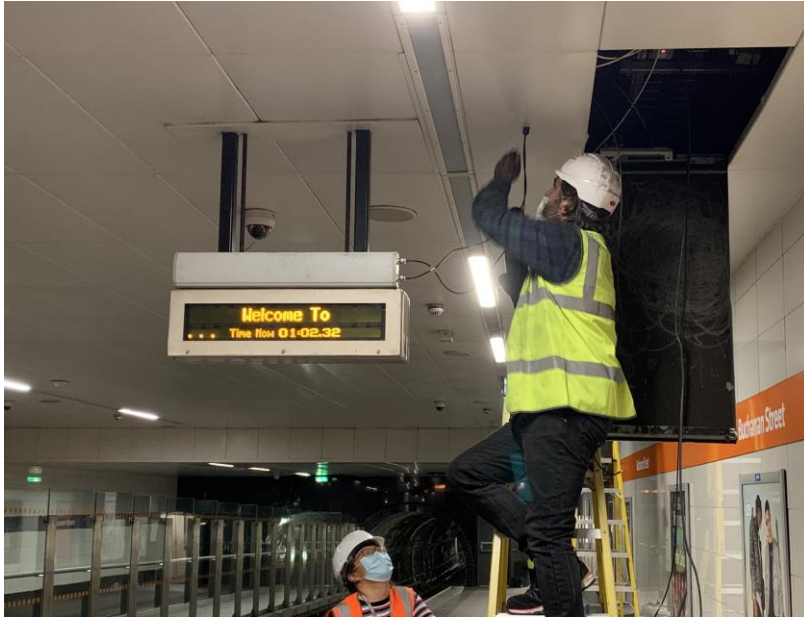
Base station antenna placed above information sign
